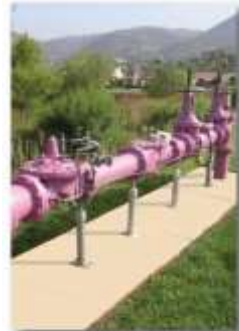
Pressure Reducing with Cavitation Protection - Reclaimed Water System
