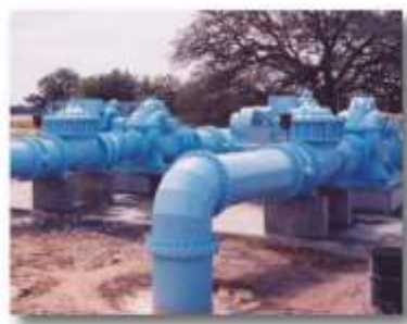
30-Inch Pump Control Valves
